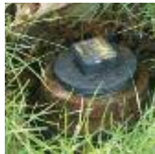
Cleanout sanitary sewer line access
