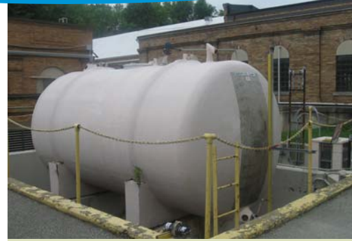
Outdoor tanks like this will be eliminated by the construction of new chemical feed buildings, which will improve safety and storage.
