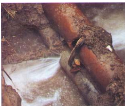
Leaking sewer lines threaten potable water supplies.
