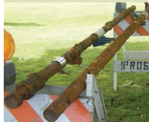
70-year old, 2-inch water main that was replaced due to its age and condition with new 6-inch and 8-inch water main.
