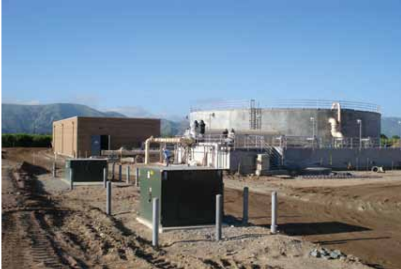
Exterior photo of the recycled water storage tank.
