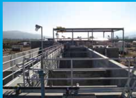
The foam and aeration basins water passes through before it reaches the membrane tanks.
