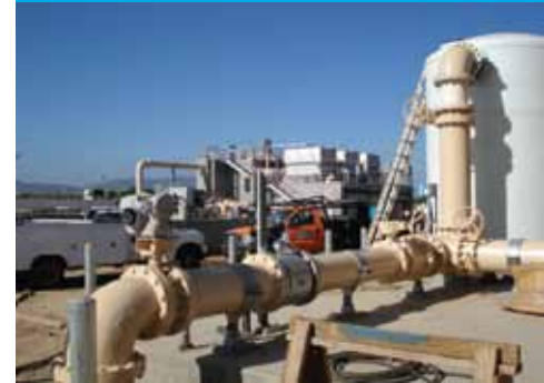
Exterior pipes feeds water to the treatment plant.
