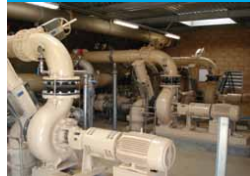
Interior photo of the plant's pump house.
