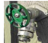
Hose bib with vacuum breaker installed
