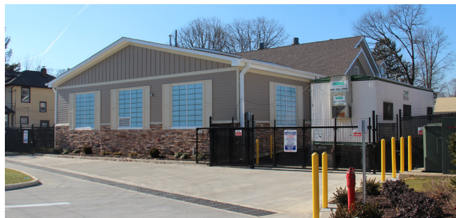
New York American Water owns 14 iron removal treatment plants statewide. The newest one (pictured here) is located in South Hempstead.
