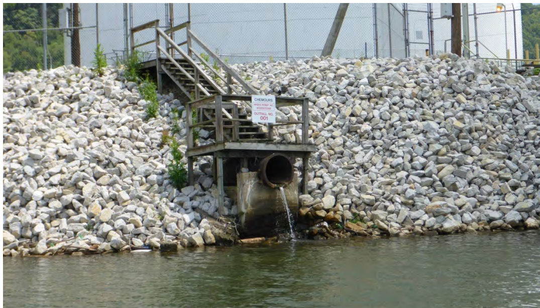
Figure 21: Outfall pipe with typical riprap along the north bank at DuPont plant.
